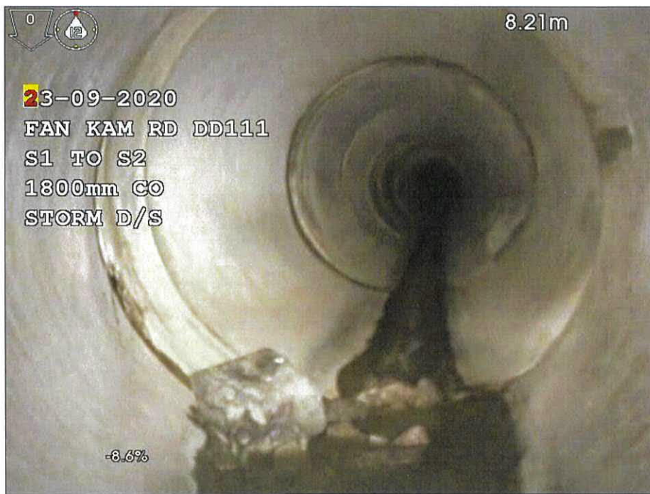
Photo Ref. : 003 Video Tape : 0001, 0:01:51 Observation : Joint Displaced Medium
