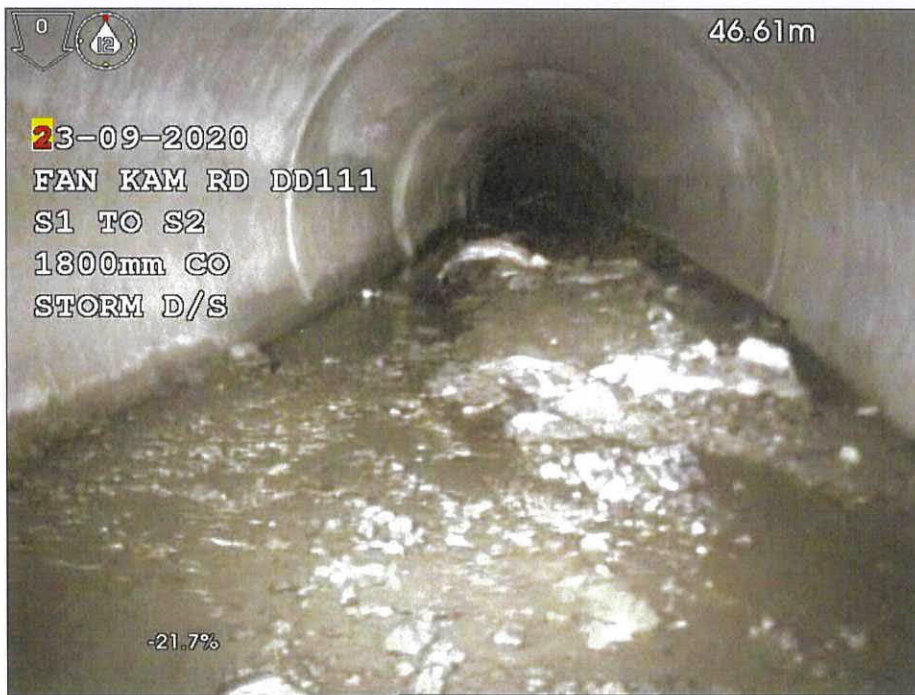
Photo Ref. : 008 Observation : Debris Silt, 35 % cross-sectional area loss, Change Video Tape : 0001, 0:04:08
