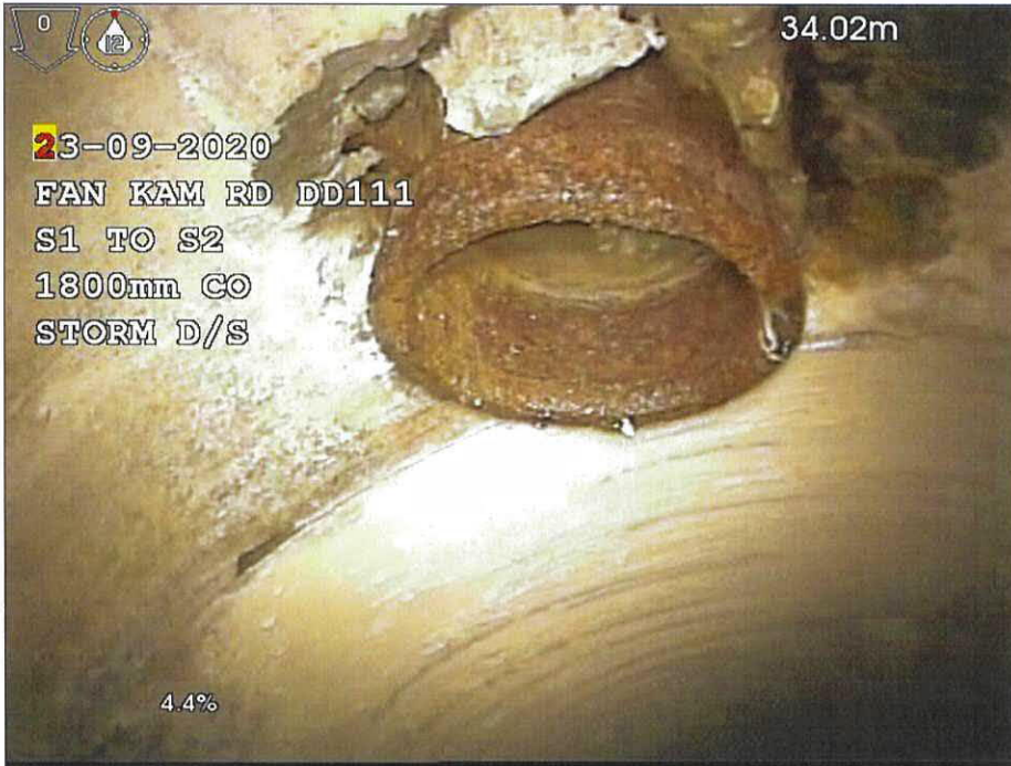
Photo Ref. : 007 Observation : Connection, at 12 o'clock, dia 150 mm Video Tape : 0001, 0:03:29
