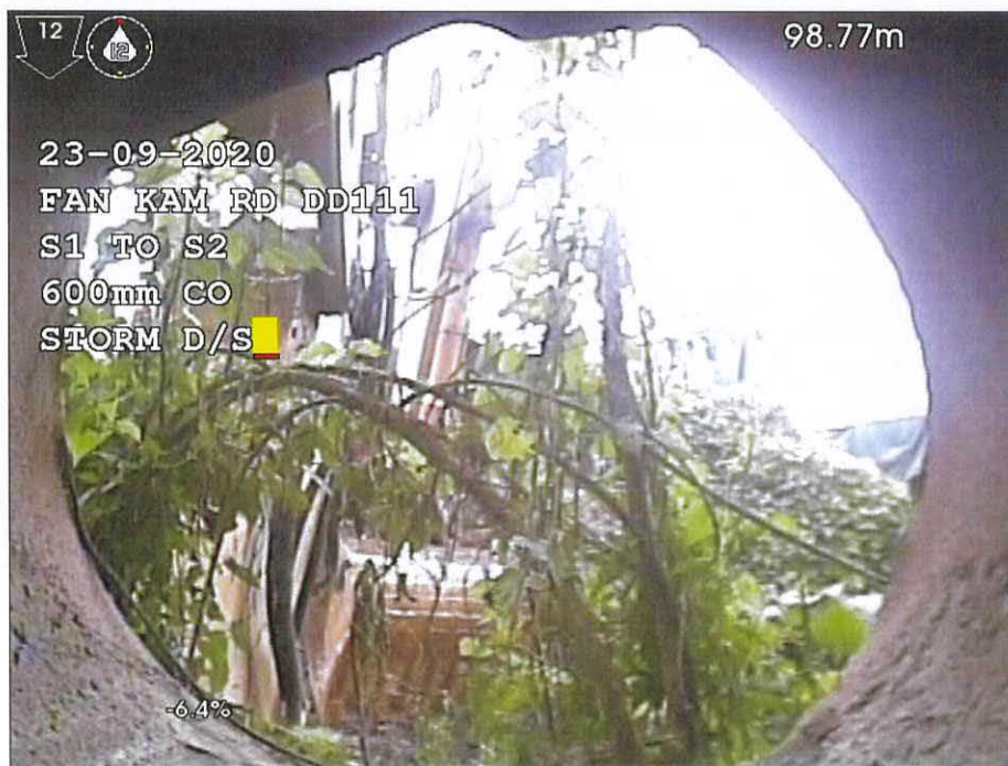
Photo Ref. : 016 Observation : Manhole Remark : S2 Video Tape : 0001, 0:10:58
