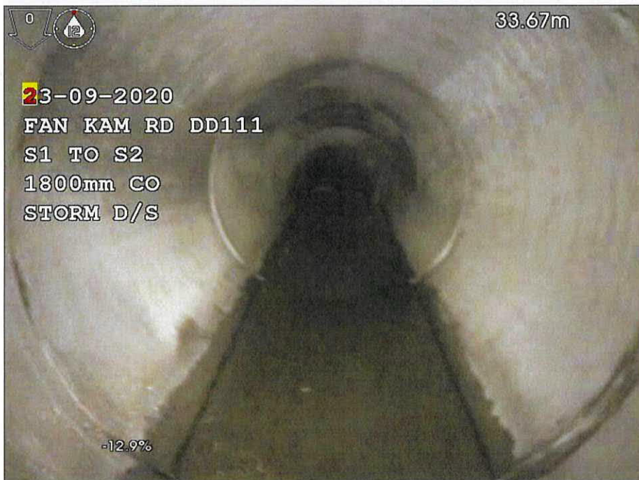
Photo Ref. : 006 Video Tape : 0001, 0:03:23 Observation : Debris Silt, 05 % cross-sectional area loss
