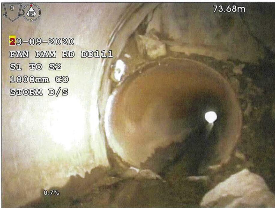
Photo Ref. : 010 Video Tape : 0001, 0:05:52 Observation : Debris Silt, 35 % cross-sectional area loss. Finish
